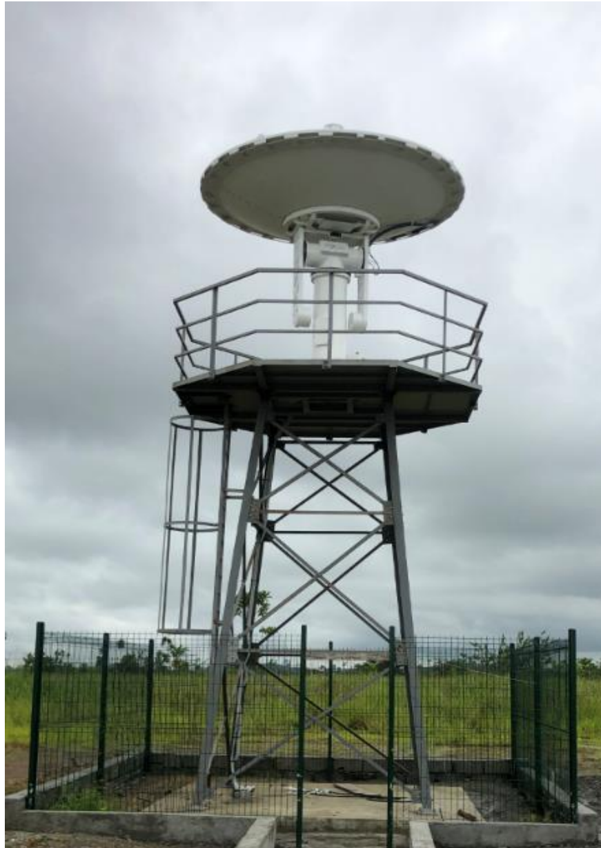
RARS station built at AGEOS's premises (Nkok- Libreville, Gabon)
